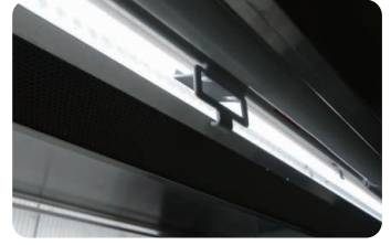
LED 조명 LED lighting
