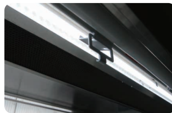
LED 조명 LED lighting
